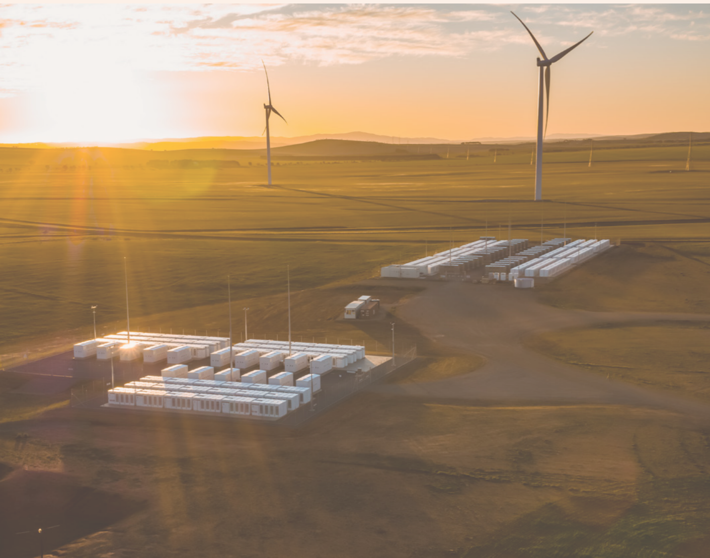
▲ Hornsdale Power Reserve and Hornsdale Wind Farm, SA. Courtesy of Neoen
