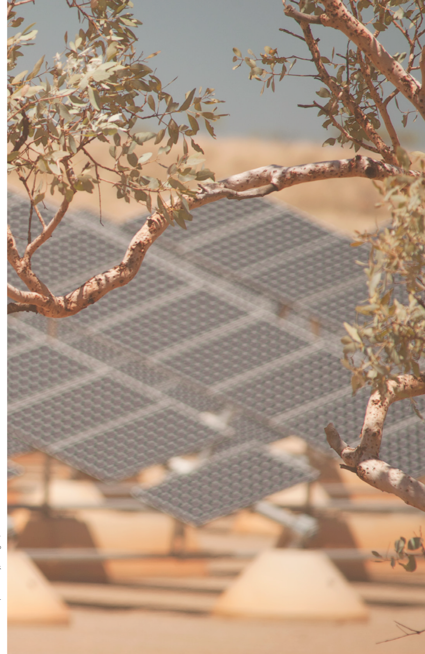
▼ Solar panel array, Nullagine, WA
