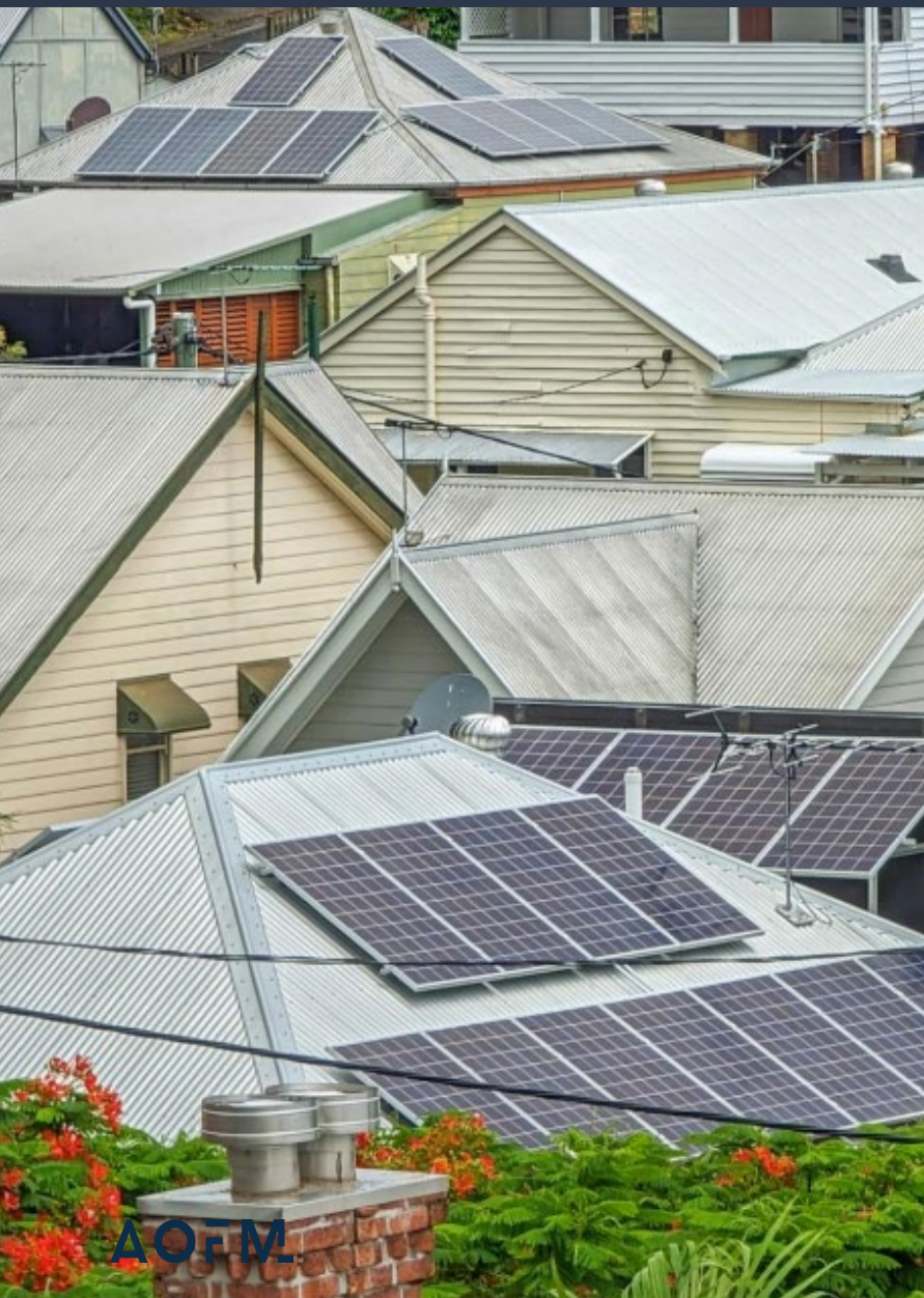
▲ Rooftop solar panels, Brisbane, QLD
