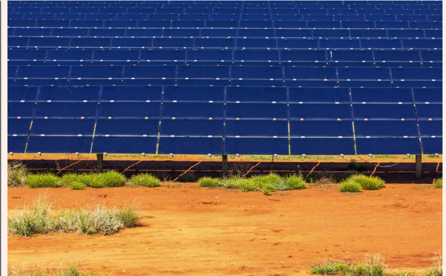
Image: Solar farm power station
