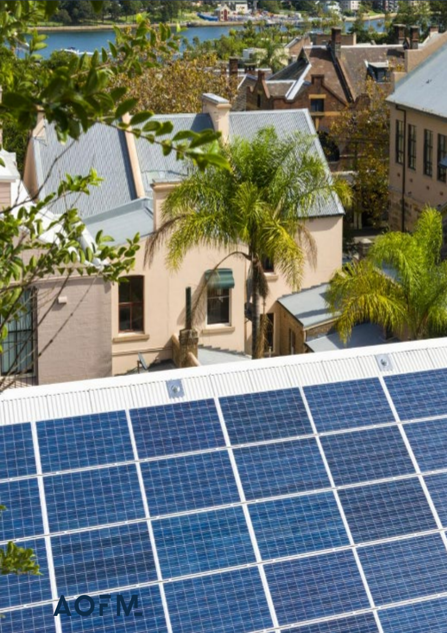
▲ Rooftop solar panels, Sydney, NSW
